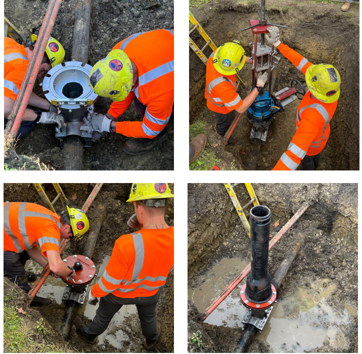
Figure 1. Many valve repair or installation projects can see significant savings by using an insertion valve rather than a traditional valve. A two-man team in the image above was to install a 4" Insta-Valve 250 in Central Illinois in about an hour.
